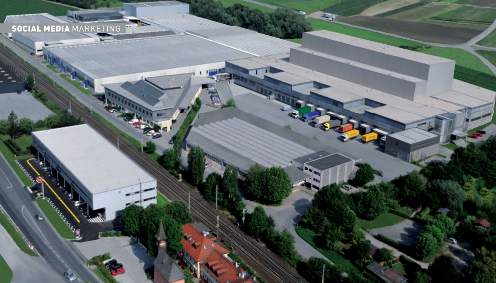
At the main production facility in Hall in Tirol, the machine manufacturer Felder has begun with the construction of a 5,100 square metre logistics centre.
