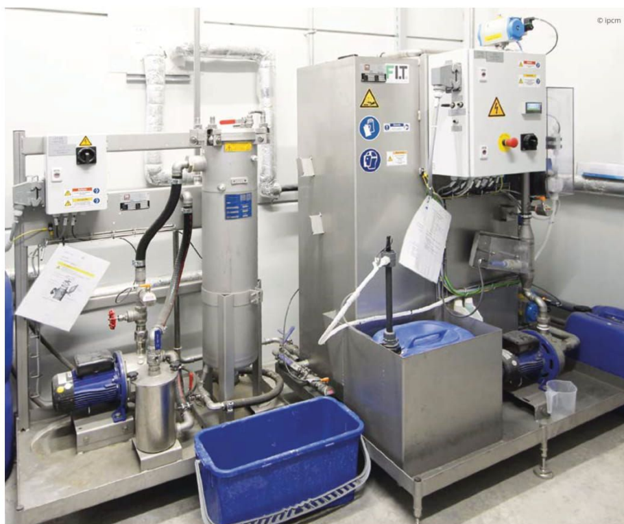
The pH control system.
