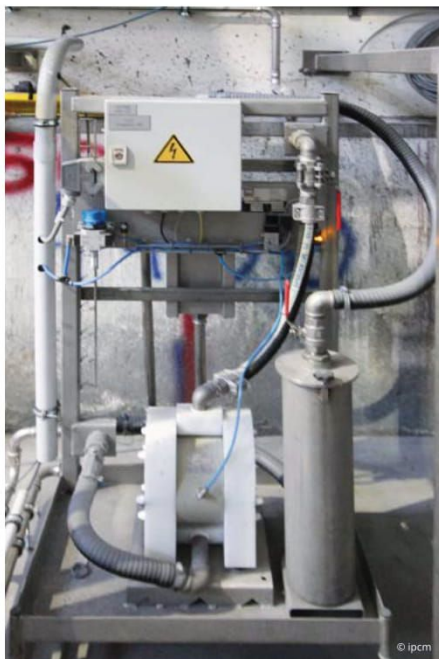
The system for sucking in water from the underground storage tank.
