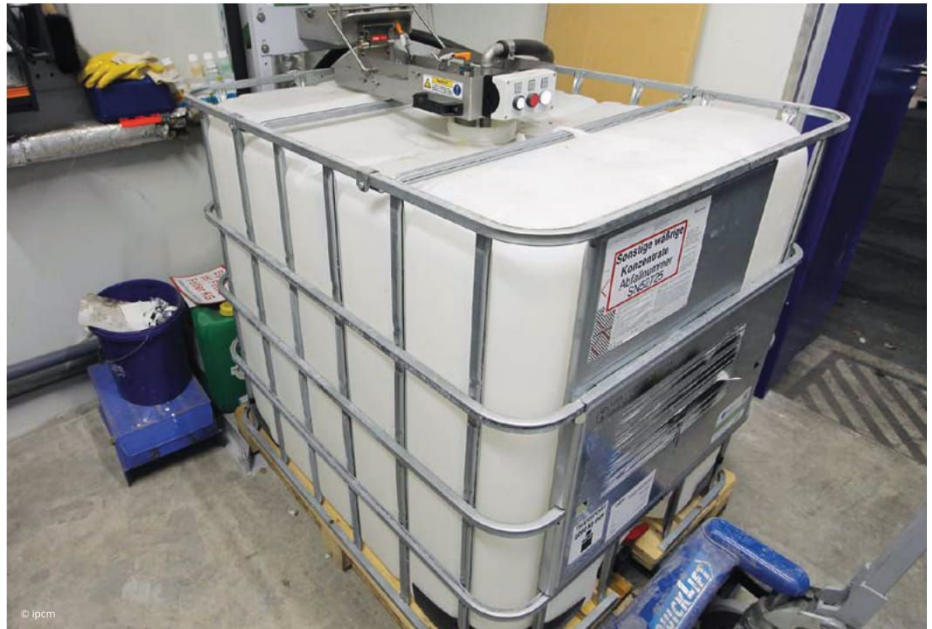
The concentrate collection tank.
