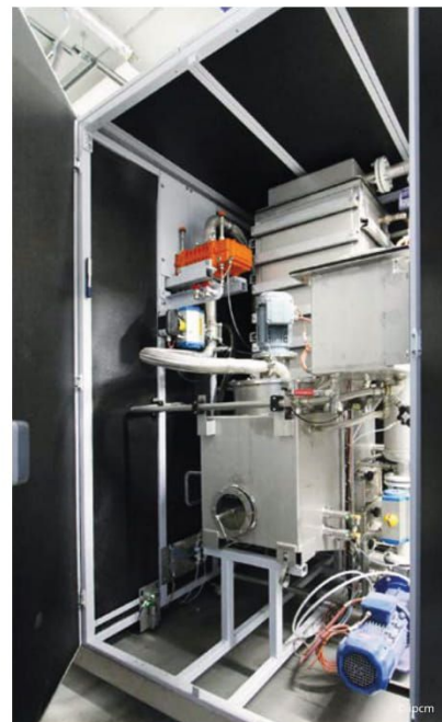
The inside of the evaporator.
